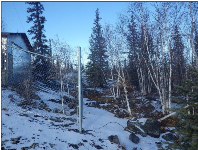
Comm Tower & Surge Raise – Inadequate Zone 1 and 2-3
