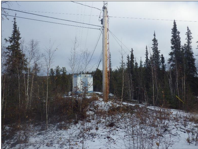
Snare Forks Radio Shack – Inadequate Zone 1 and 2-3 Clearance
