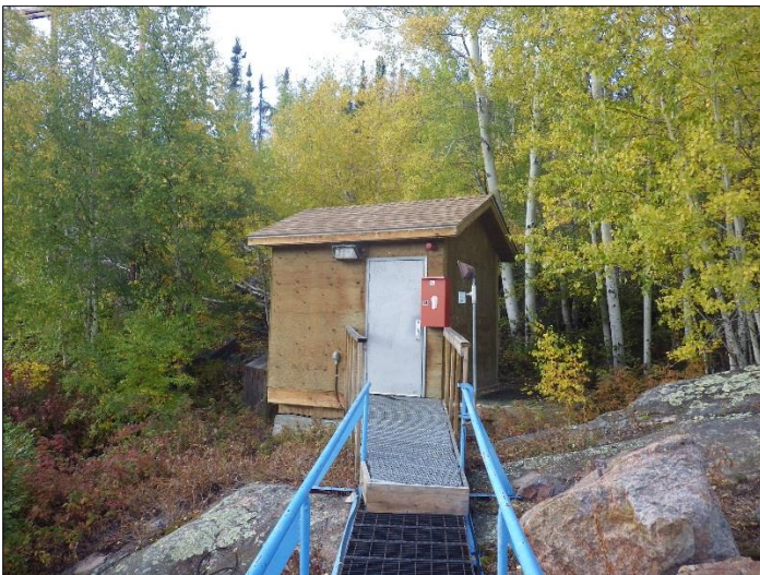
Sump Shack – Inadequate Zone 1 Clearance
