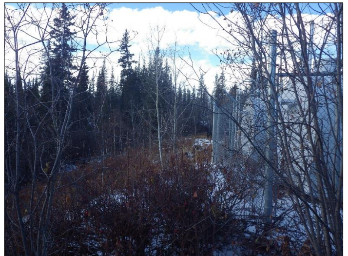
Gas Tanks – Inadequate Zone 1
