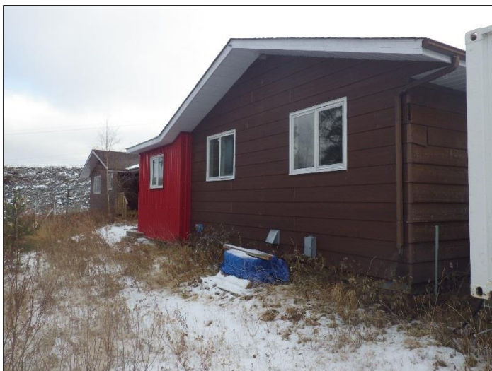
Snare Rapids Camp – Wooden Porches and Inadequate Zone 1
