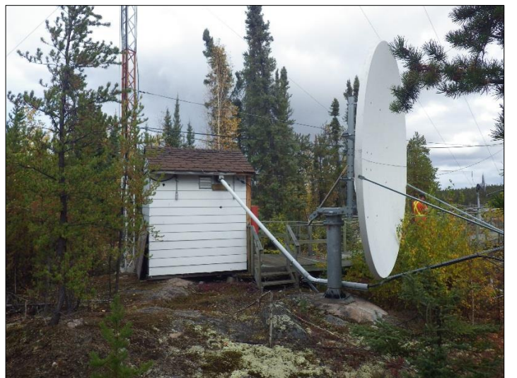
Comm Tower – Unskirted and Combustible Walkway
