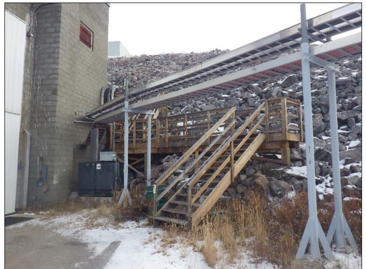
Snare Rapids Powerplant – Combustible Wooden Steps
