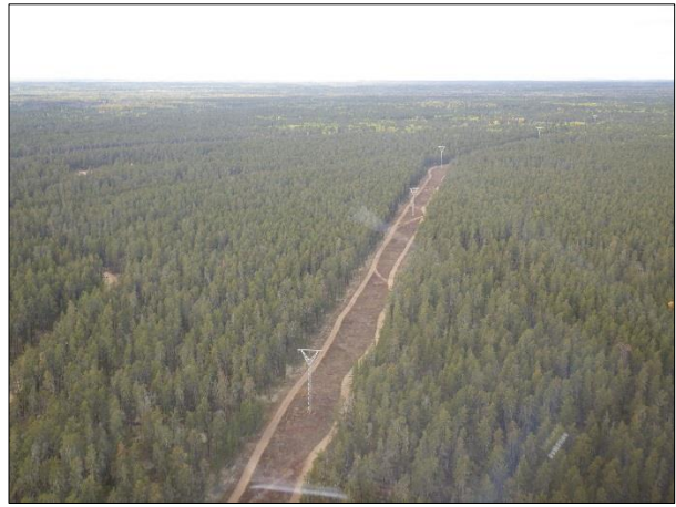
Metal Poles – Taltson to Fort Smith
