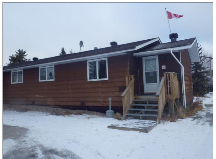
Snare Rapids Camp – Un-skirted Building and Porch Undersides
