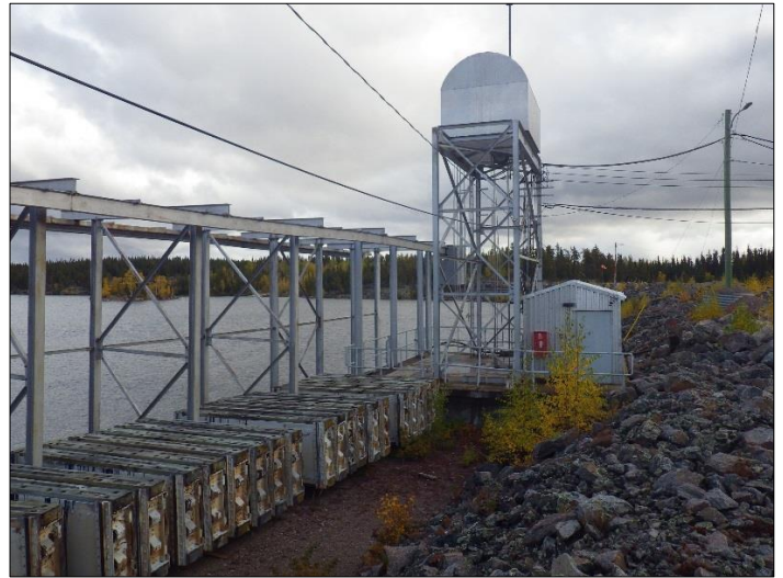
Headworks – Minimal Threat
