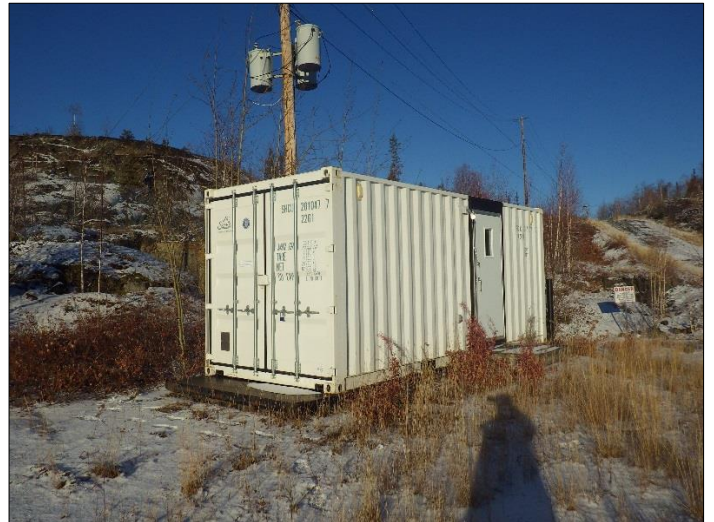
Portal Shack – Inadequate Zone 1A Clearance
