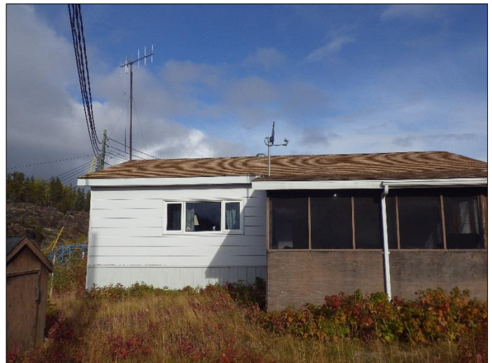
Camp – Inadequate Zone 1 Clearance from Grass/Brush
