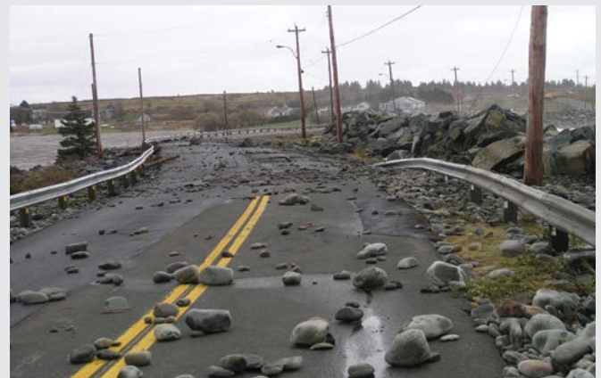
FIGURE 15: Effects of storm-wave overwash on Cow Bay Road, Halifax Regional Municipality, NS. Photo courtesy of R.B. Taylor.
