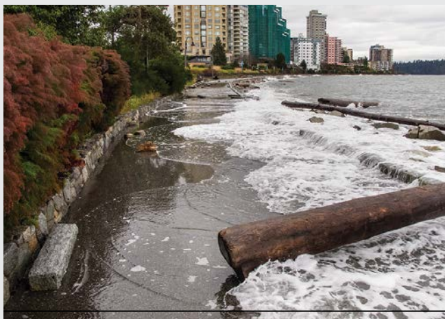
FIGURE 19: Wave damage to the West Vancouver seawall during a storm. Photo courtesy of the West Vancouver Shoreline Preservation Society.
