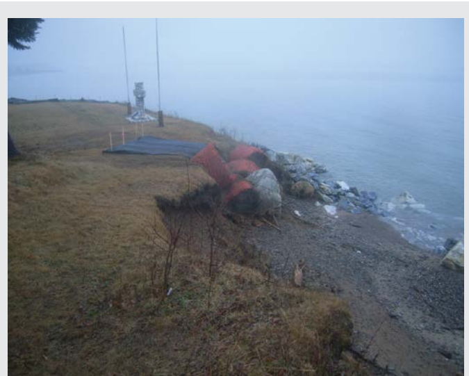
FIGURE 15: Malagawatch Cemetery, NS, where buried human remains eroded into the sea following several storm events. Initial protection of the site involved the use of stone armoring (as seen below the cross). Subsequent storms and erosion led to temporary protection of burials using anchored hay bales and a permeable membrane (centre of photo). Planning for more permanent protection is ongoing. Photo courtesy of Heather MacLeod-Leslie.
