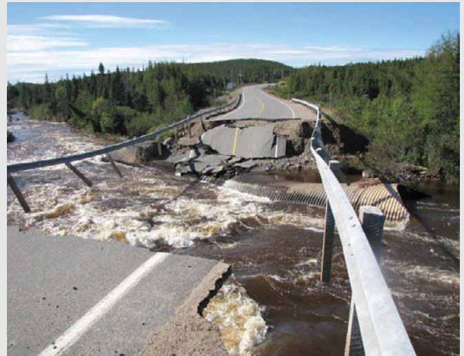
FIGURE 4: Washout of highway and bridge near Port Rexton, NL. Photo courtesy of Fire and Emergency Services, Newfoundland and Labrador.
