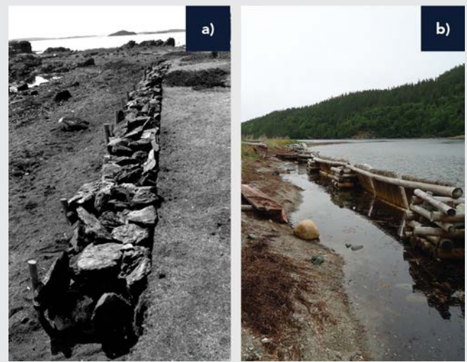
FIGURE 16: Two different construction methods used to protect archeological sites in Bonavista Bay, NL: a) the stone gabion wall constructed at Inspector Island (Pastore, 1987) has successfully protected the site for three decades; b) wooden breakwaters have consistently failed at the Beaches site. Photo b) courtesy of Anita Johnson-Henke.
