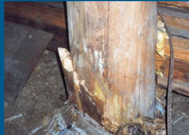
Total Pile collapse at Ground level.
