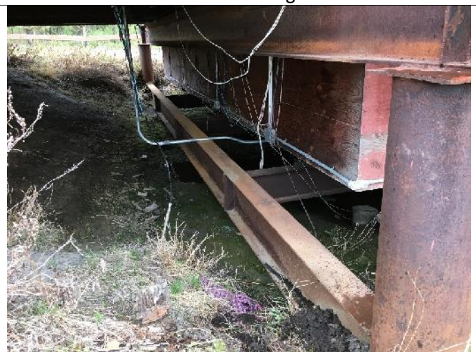
Low spot under middle of building with standing water
