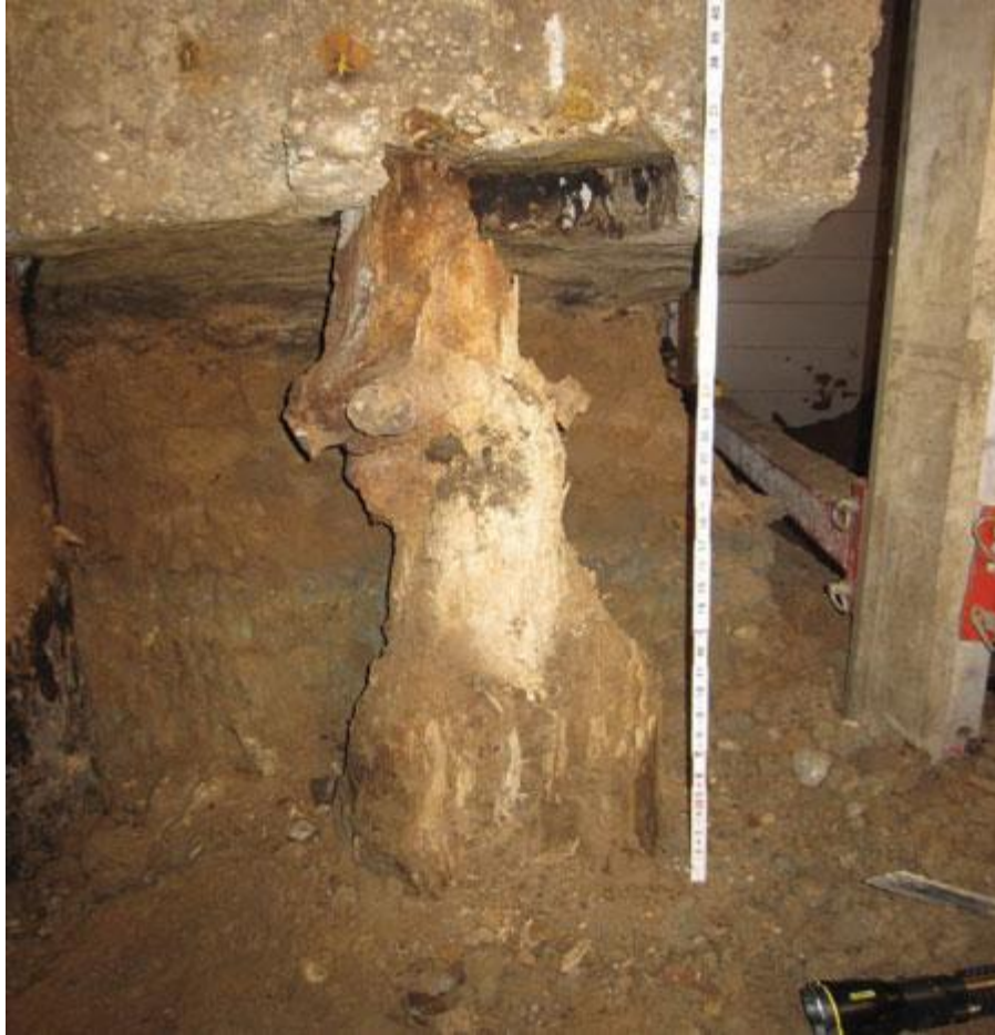
Figure 3. Example of severely decayed timber pile below concrete pile cap at Test Pit No. 1
