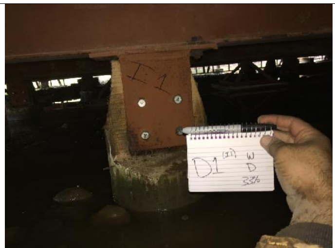
D3 – Incorrectly labelled as D1
