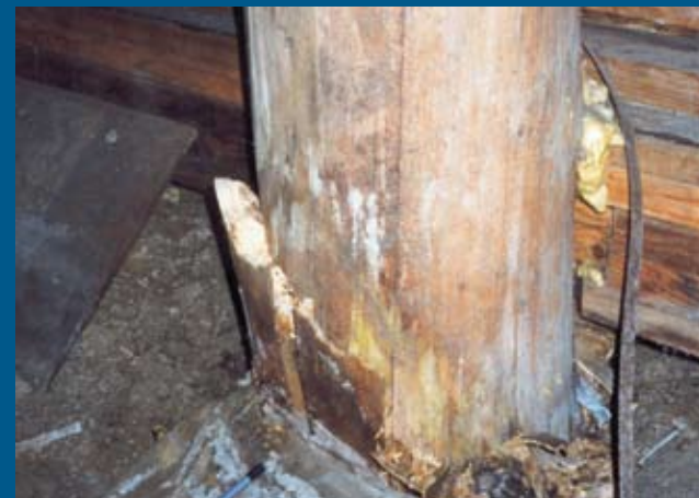
Total Pile collapse at Ground level.
