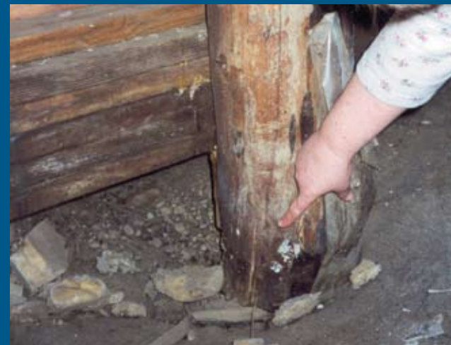
Depression holds water around pile, speeding up rot.
