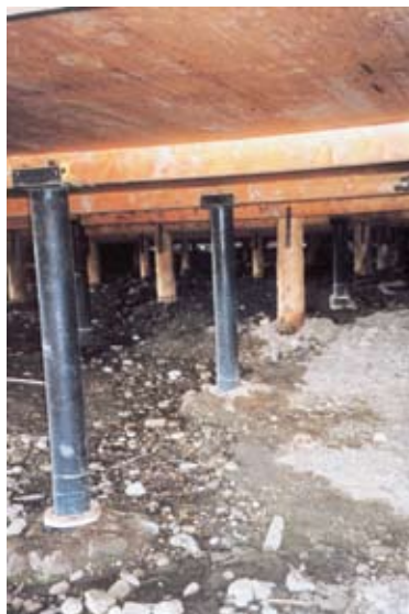
New steel posts connect solid piles below the earth to the building.
