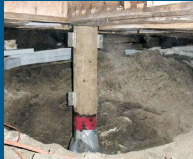
The rotted portion of this pile has been replaced with new material.
