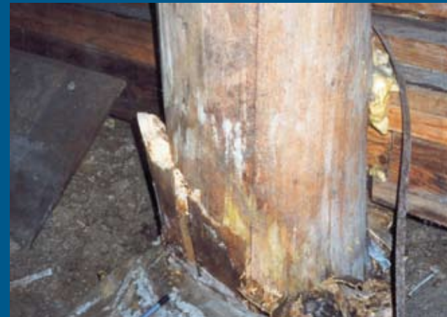
Total Pile collapse at Ground level.
