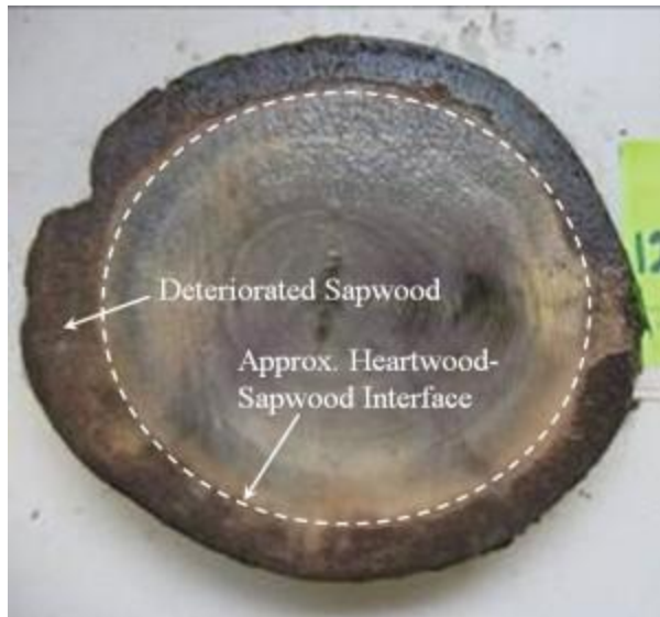
Figure 1: Deteriorated timber pile cross-section.
