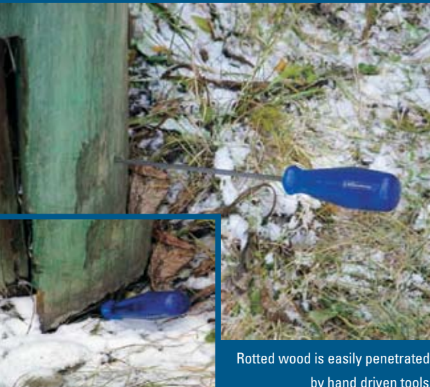
Hand tool used as probe to locate soft pile rot.
