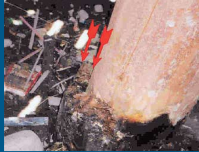
Total pile collapse and shift at ground level.
